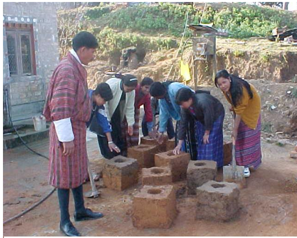
Village women constructing the chimney for fuel-efficient stoves during Capacity Building Training. Also seen in the picture is a technician from MTI
